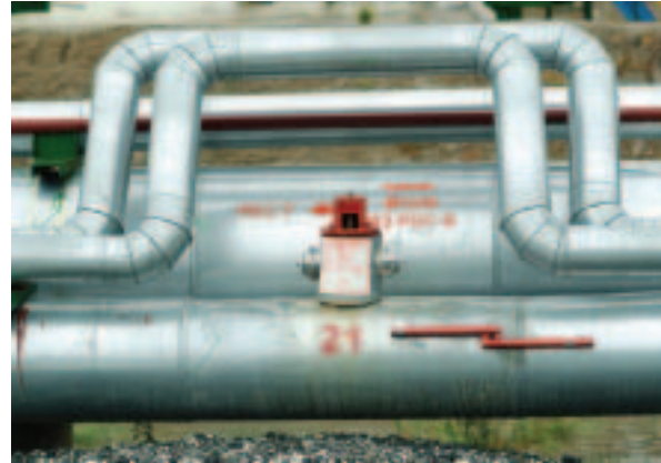
WATER PIPELINES AT SLYM
