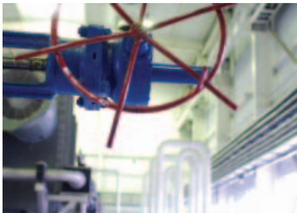
INSIDE THE SALYM PUMP HOUSE
