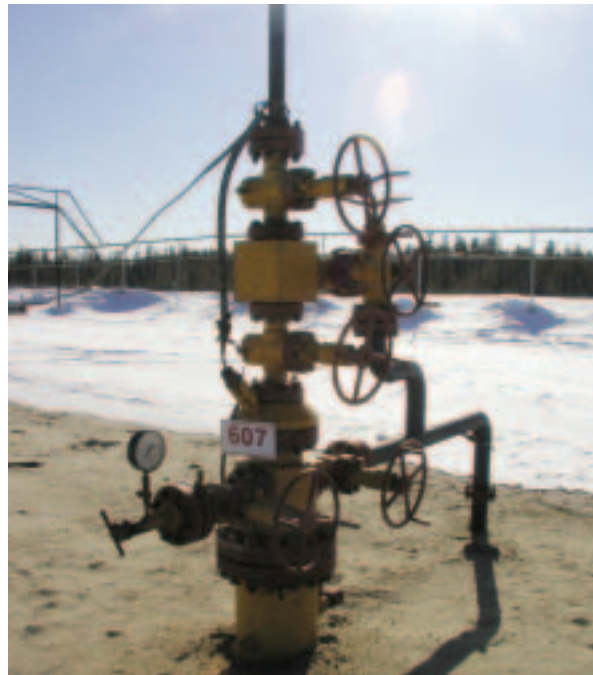
Above: Well head at the Yuzhnoe Oil Field (Magma)
