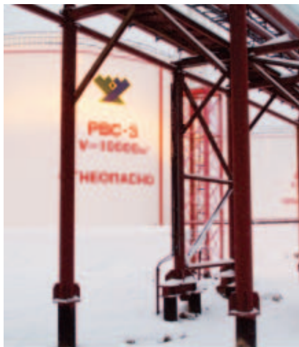
Above: 10,000 m 3 storage tanks at Salym CPF
